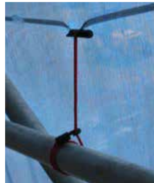
POWERCLAD FTFR TIED TO THE SCAFFOLD STRUCTURE, WITH A POWERTIE. NOTICE THE SHORT DISTANCE BETWEEN THE TYING LOOPS.
