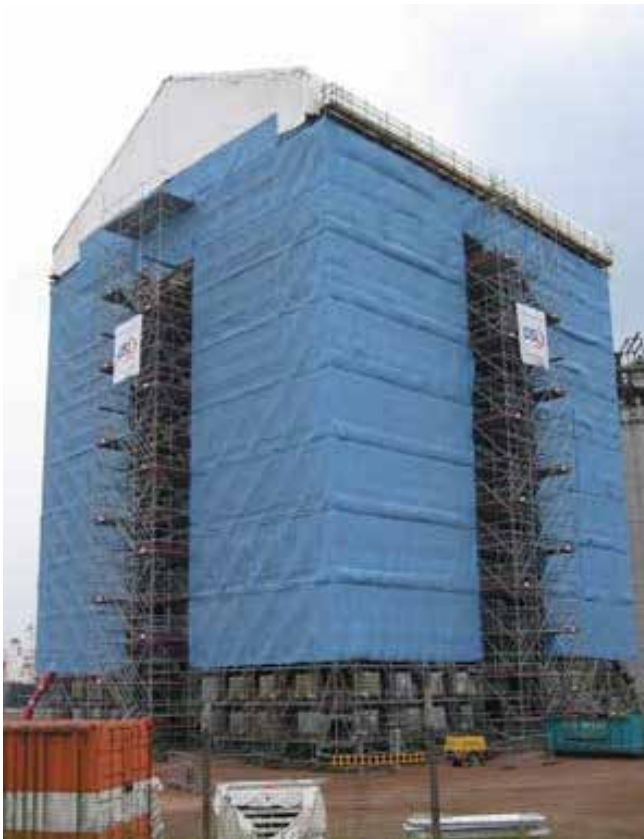
PETROCHEMICAL STORAGE TANK ENCAPSULATED WITH POWERCLAD FTFR.
